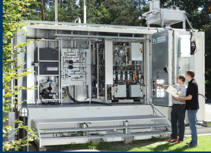
Test bench: 1 MWh LOHC storage system
