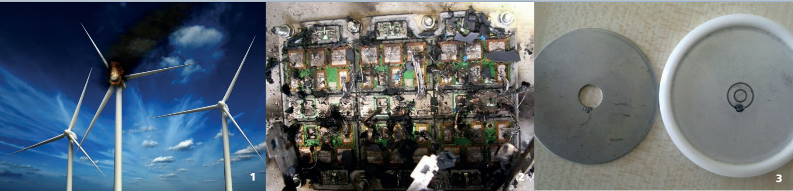
1 - 3 Examples of power electronic damages
