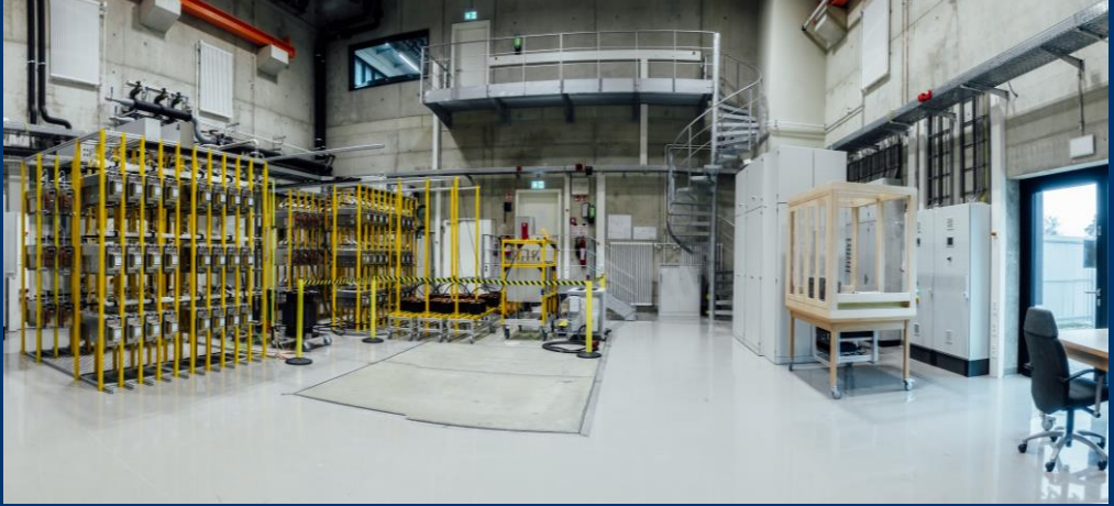
Fraunhofer IISB Medium Voltage Test Bench – Innovative test infrastructure for future grids
